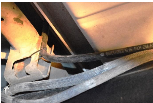
(Fig. 9) One of the vent hoses routed up and attached to the vehicle's body with quick tie.
